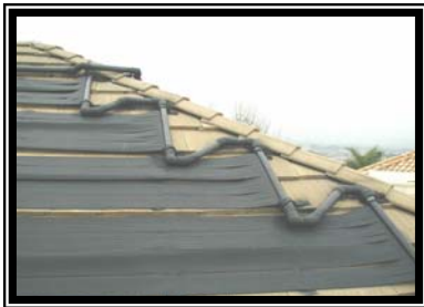
Connecting the headers of a staggered system.
